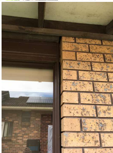
Gap between brickwork and window suggest foundation movement
